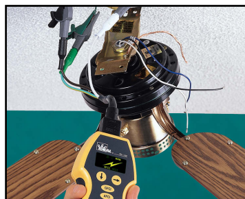
AFCI testing with alligator clips on an installed device.
